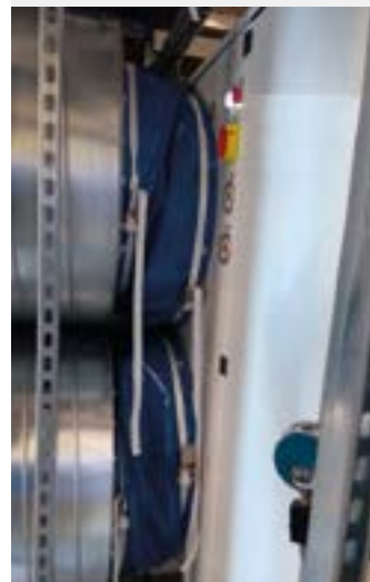
High pressure fan.
